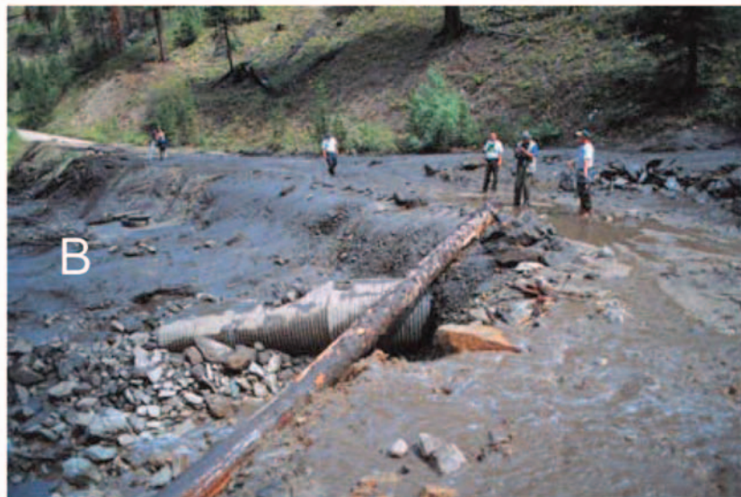
Figure 16 —Water repellent soil layers (A) after wildfires can promote soil erosion (B), which in turn can impact domestic water supplies, decrease site productivity, and slow vegetative recovery (K. Watenmaker photos).
